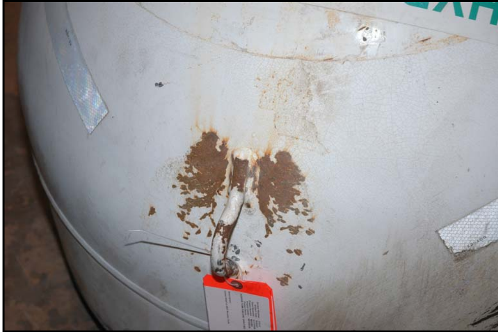
Figure 7: Shows corrosion on the tank head.
