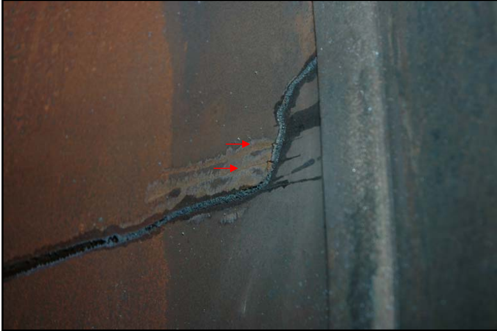
Figure 5: Two cracks (indicated by arrow) observed parallel to the fracture surface on the ID of the tank head.
